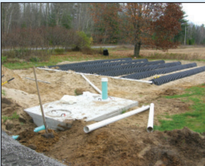
Leaching bed with gravelless trench technology.
